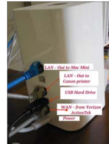
Figure 3. The cable arrangement on my Airport Extreme.
